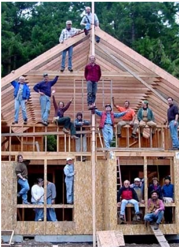
Innisfree LEC, Lopez Community Land Trust (Lopez Island, WA) Residents help build their future homes as part of their sweat equity requirement.
